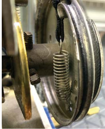
Figure 29. Capacitor control close-up.
