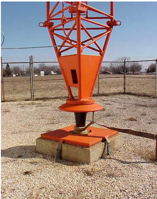
The ceramic insulator at the base of the tower. Note the rectangular hole in the faceplate.
