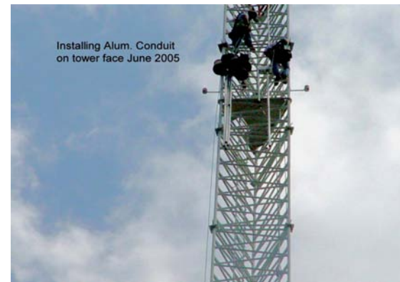
The "platform" and side light system can be seen here during a retrofit of the tower.
